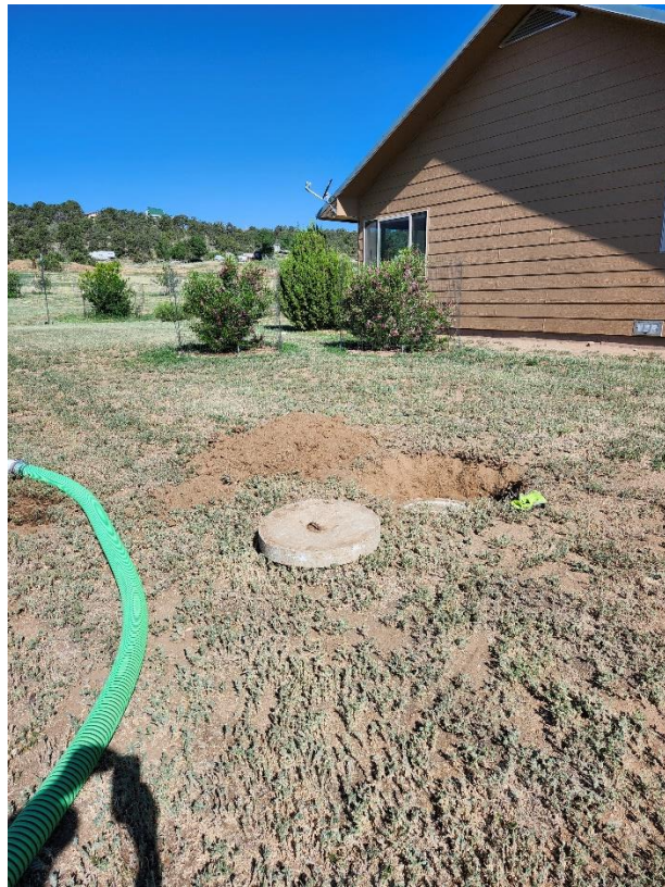
View of south chamber riser looking towards the SE corner of the home. The sewer line runs from the SE corner of the home to this south chamber of the septic tank.
