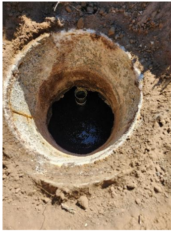
Effluent baffle, north chamber
