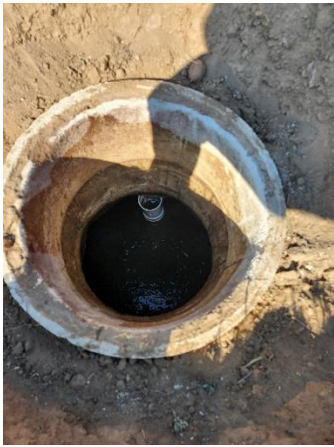
Influent baffle, south chamber
